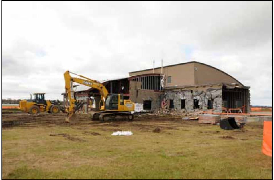
Construction is underway on the fire station to make it much more energy efficient building, providing an energy cost savings of an estimated 30 to 60 %. Photo by Tech. Sgt. Dan DiPietro
